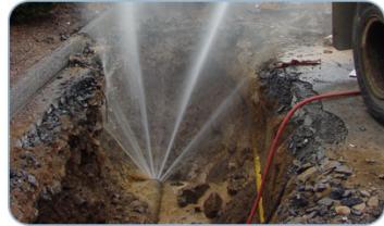
A leaking water main
