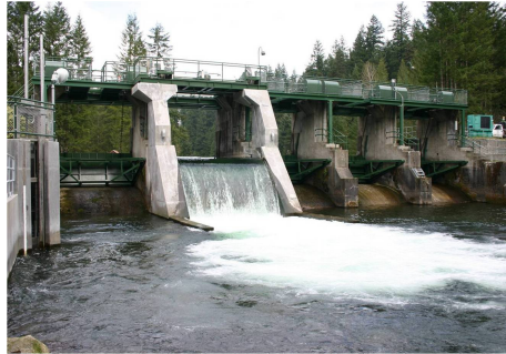
Landsburg Diversion Dam
